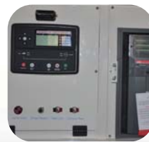
Control Panel & MCB
